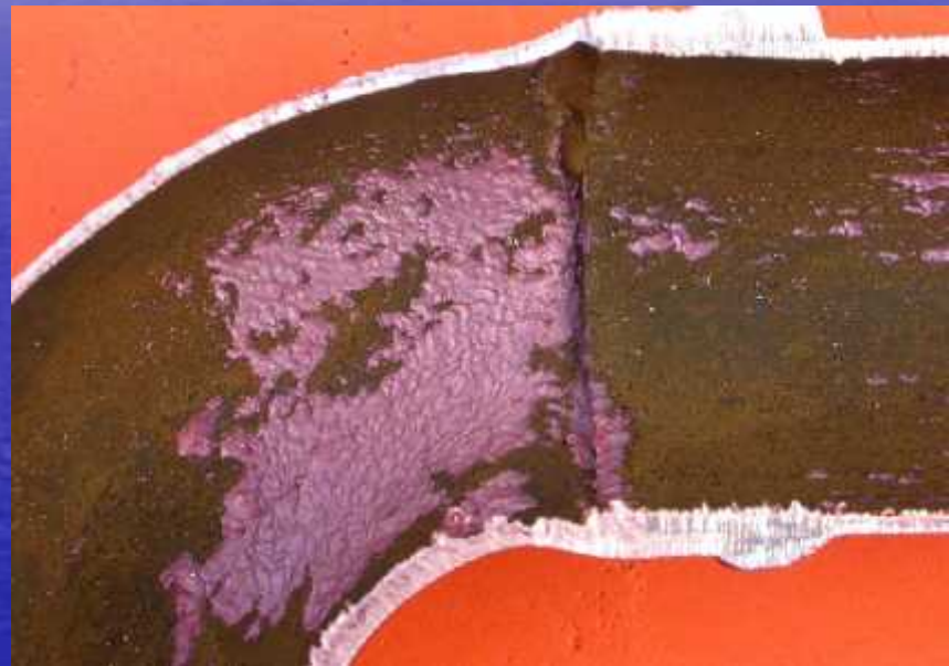
Erosion-Corrosion downstream of a joint, apparently due to turbulence at the joint.
