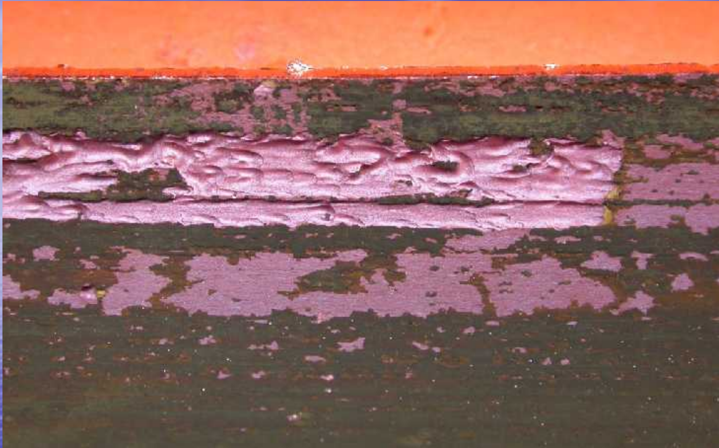
Early stages of Erosion-Corrosion attack. Horseshoe-shaped pits have open end downstream.
